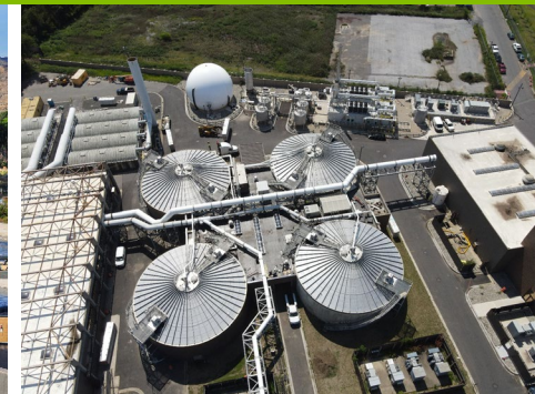
CAMDEN COUNTY MUNICIPAL UTILITIES AUTHORITY CAMDEN, NJ SUPPLY + O&M
